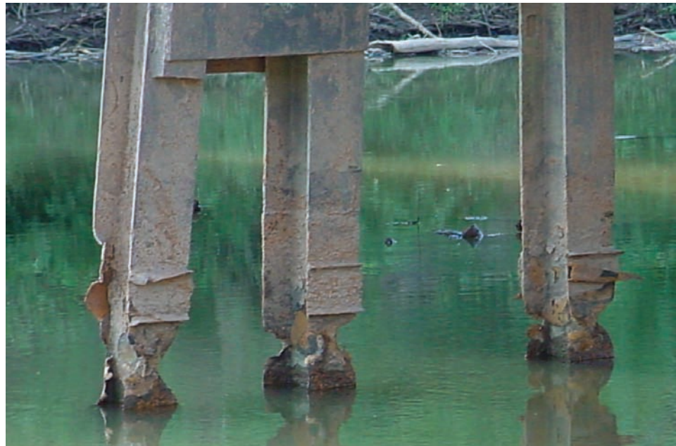
Figure 11.3.28 Deteriorated Steel Piles at Splash Zone
