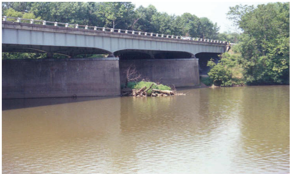
Figure 11.3.13 Buildup of Debris At Pier
