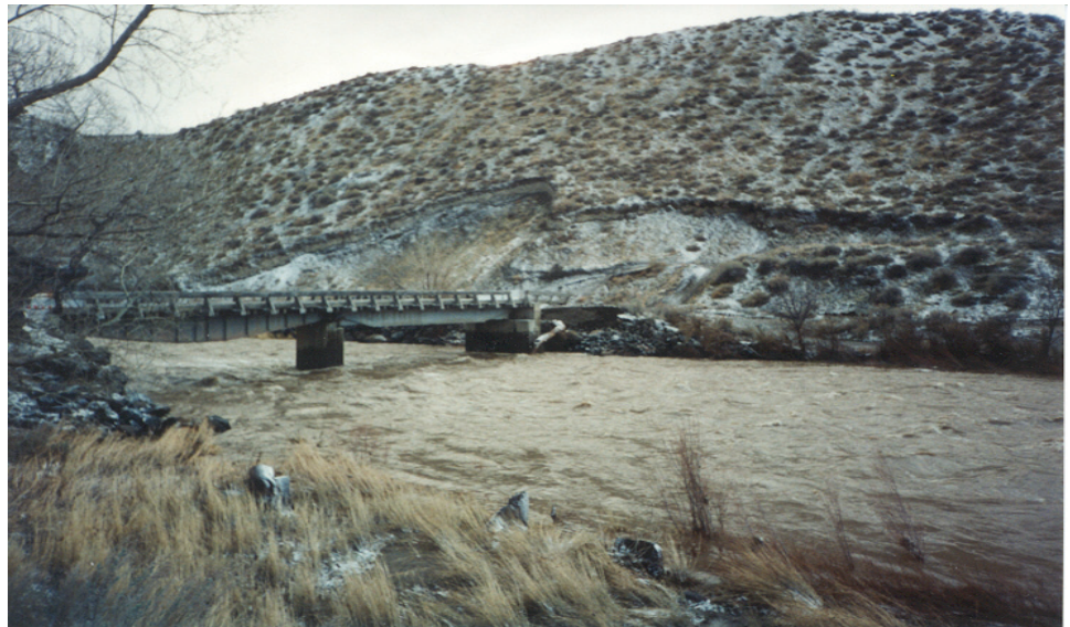
Figure 11.3.21 Severe Flood-Induced Abutment Scour
