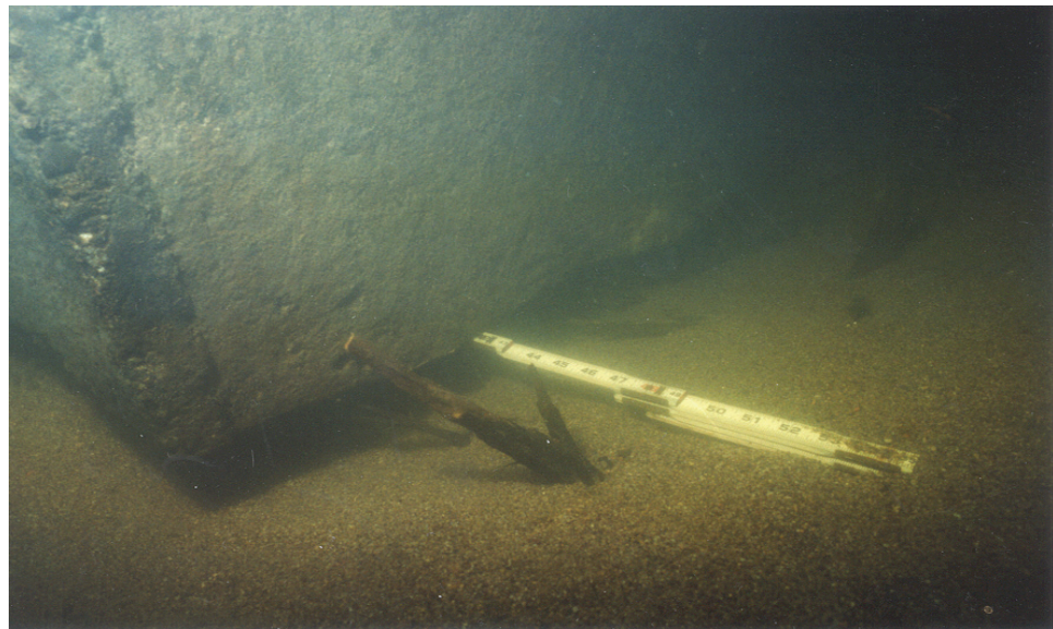
Figure 11.3.11 Local Scour; Causing Undermining of a Pier
