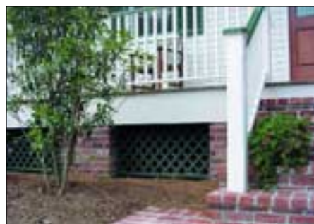
The ground beneath an open pier-and-beam foundation should be graded to provide drainage away from the structure.
