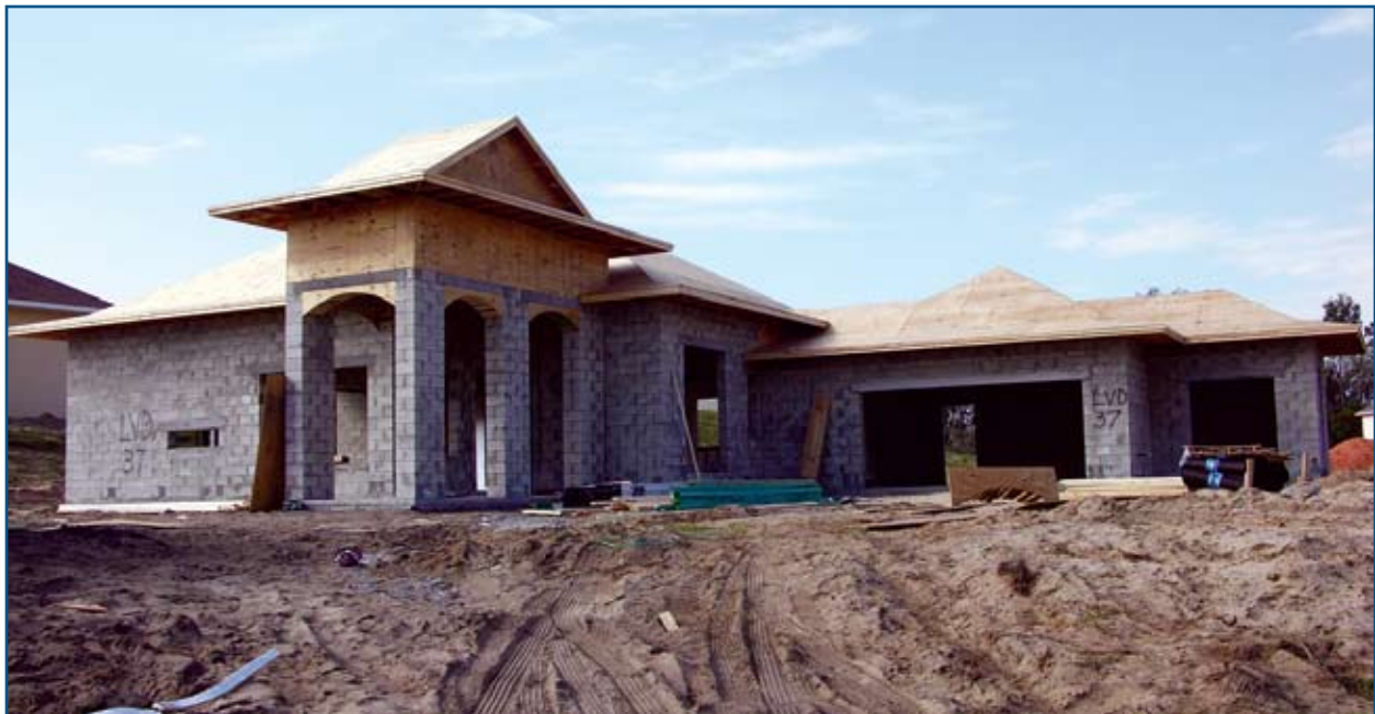
Figure II-5. CMUs were used for the exterior walls at this home under construction (New Smyrna Beach, Florida).
