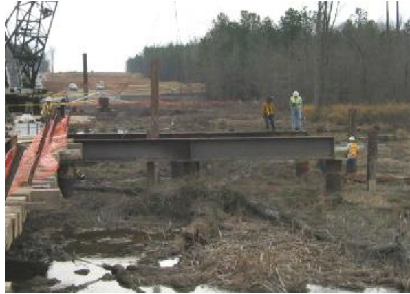
Figure 27 Steel pipe piles, steel pier caps, and steel framing, with a timber mat deck, form the structural system for this temporary work bridge.
