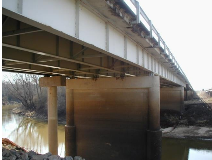
Figure 31 Example of the wide range of variations in pier types. This project featured the widening of an existing bridge which used multi-column piers with web walls. The widened section used single column hammerhead piers.
