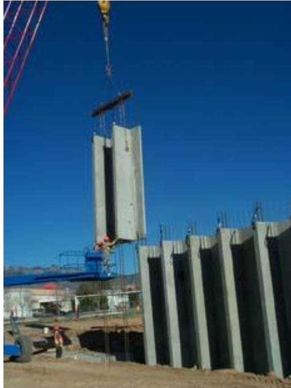
Figure 33 Opportunities abound for innovation in substructure design. This unique full height abutment which uses precast double-tees for the stem wall is one example of a creative solution that addressed the specific criteria of a given project.
