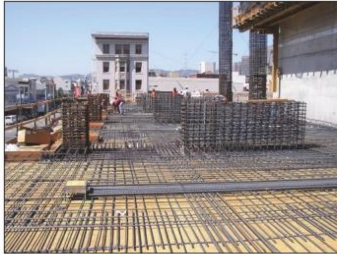
Figure 33. Conflict between the location of collector reinforcing with a nonstructural component.
