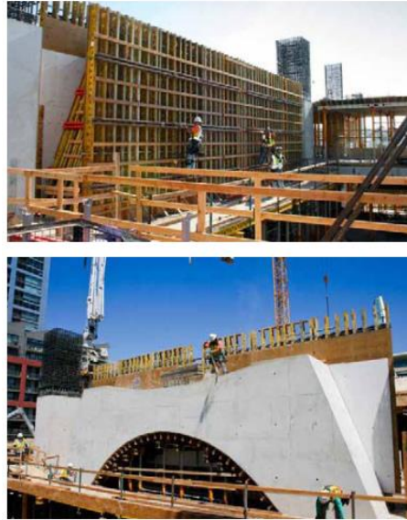
Figure 9. Gravity Arch Supports San Diego Library
