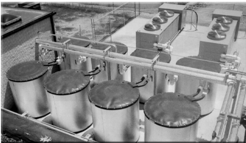
Modular ice-on-coil storage tanks with condenser units above
