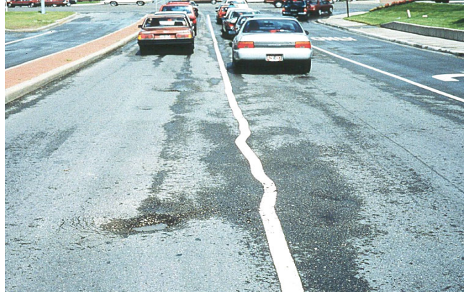
d) Drainage problems
