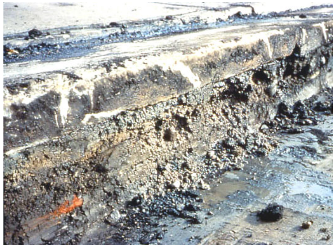
b) Aggregate contamination or degeneration
