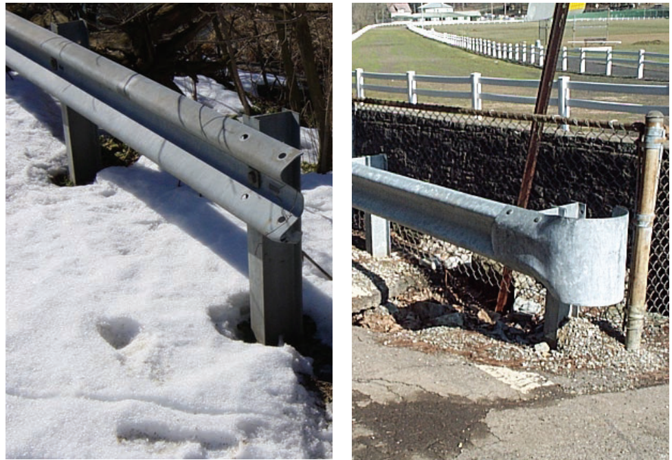
Figure 5.5.9 Unacceptable Blunt Ends
