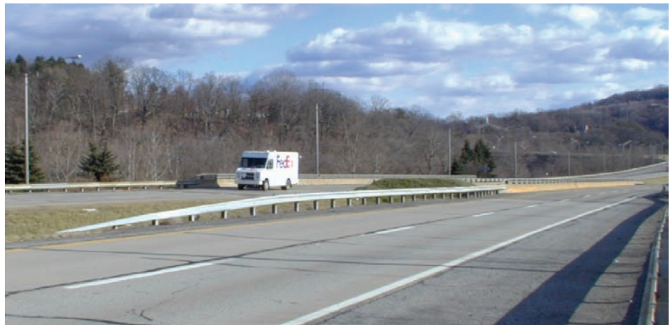
Figure 5.5.3 Bridge Railing, Transition, Approach Guardrail and End Treatment (Turn down end treatment no longer acceptable for this roadway type)
