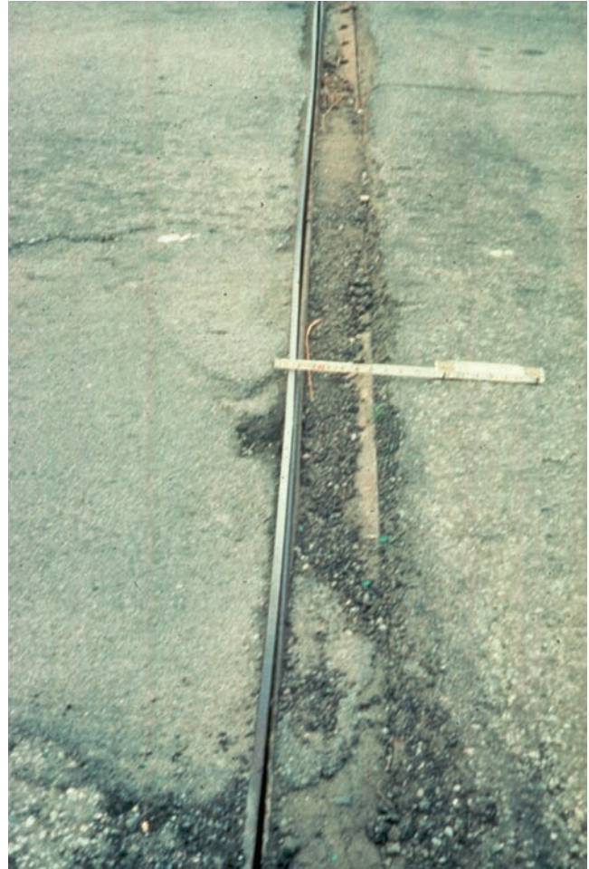
Figure 5.4.15 Debris Lodged in a Sliding Plate Joint
