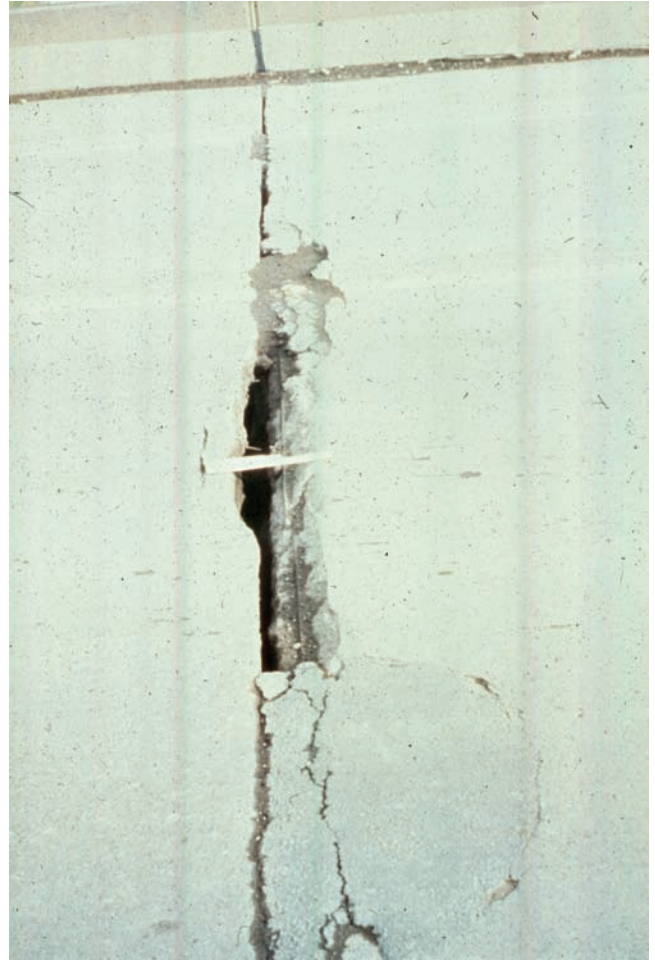
Figure 5.4.18 Failed Compression Seal
