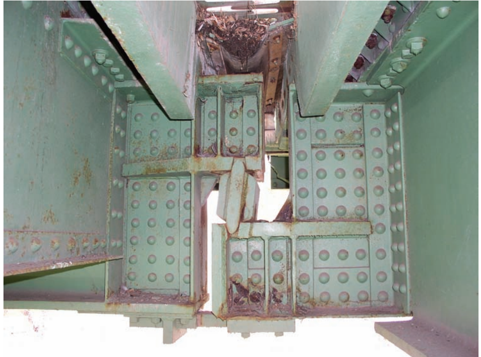
Figure 5.4.22 Drainage Trough with Debris Accumulation
