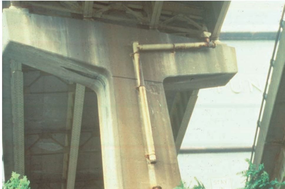
Figure 5.4.14 Downspout Pipes and Cleanout Plugs
