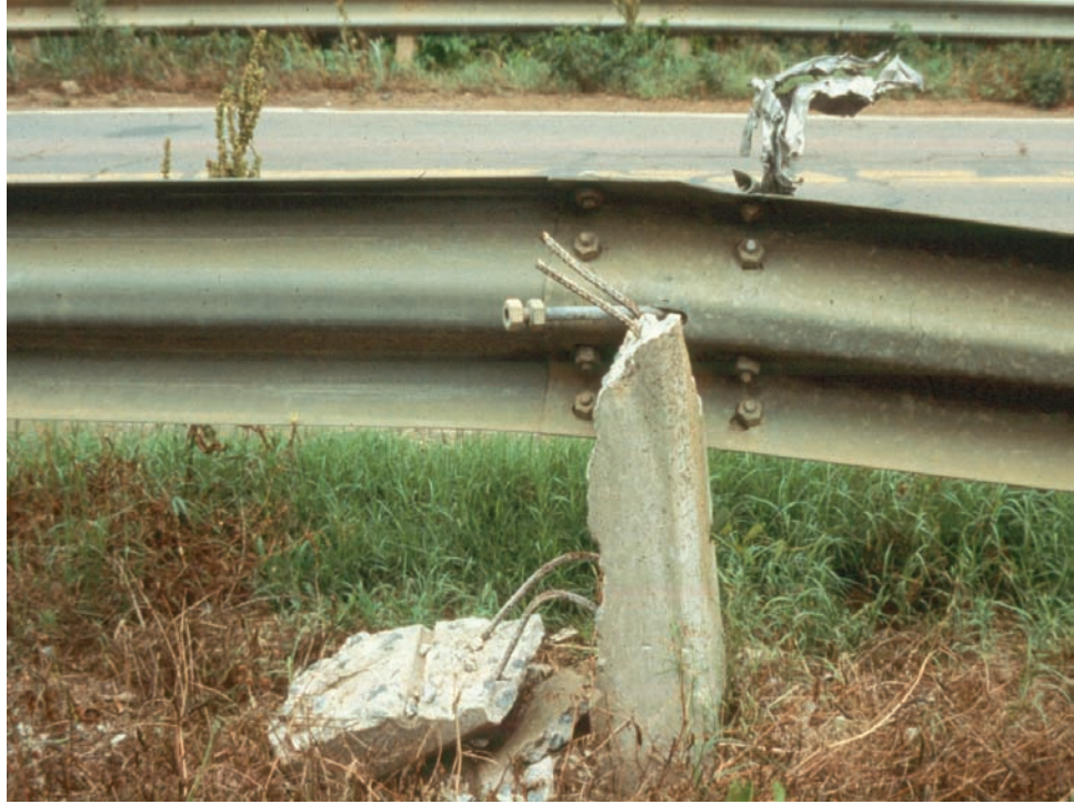
Figure 5.5.11 Approach Guardrail Collision Damage
