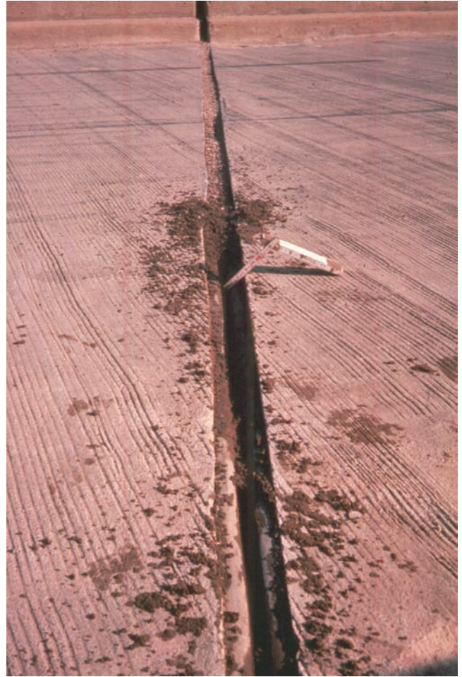
Figure 5.4.16 Dirt in a Compression Seal Joint
