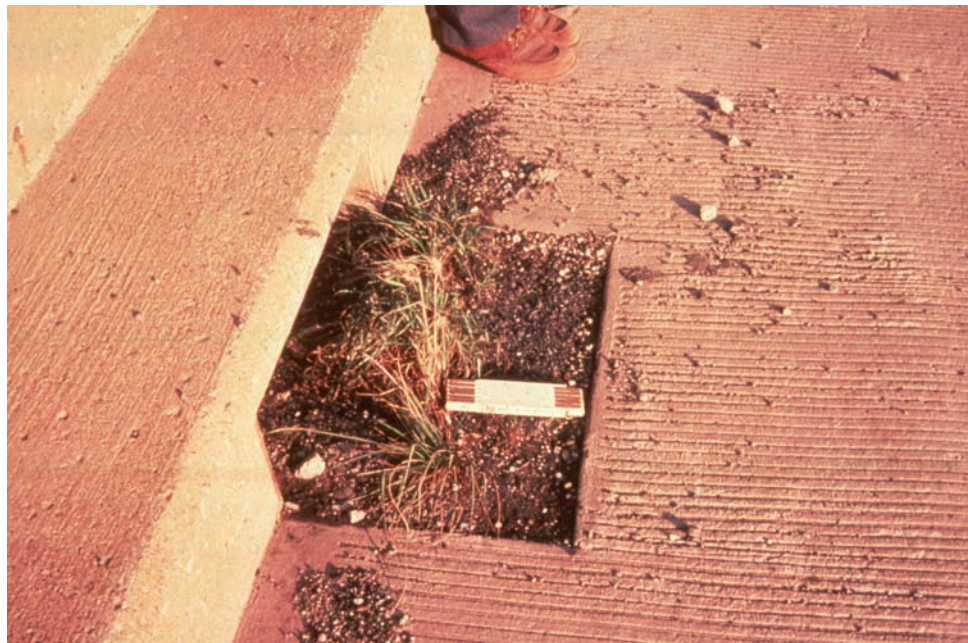
Figure 5.4.21 Clogged Drainage Inlet
