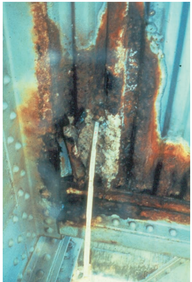
Figure 5.2.12 Deteriorated Stay-in-Place Form
