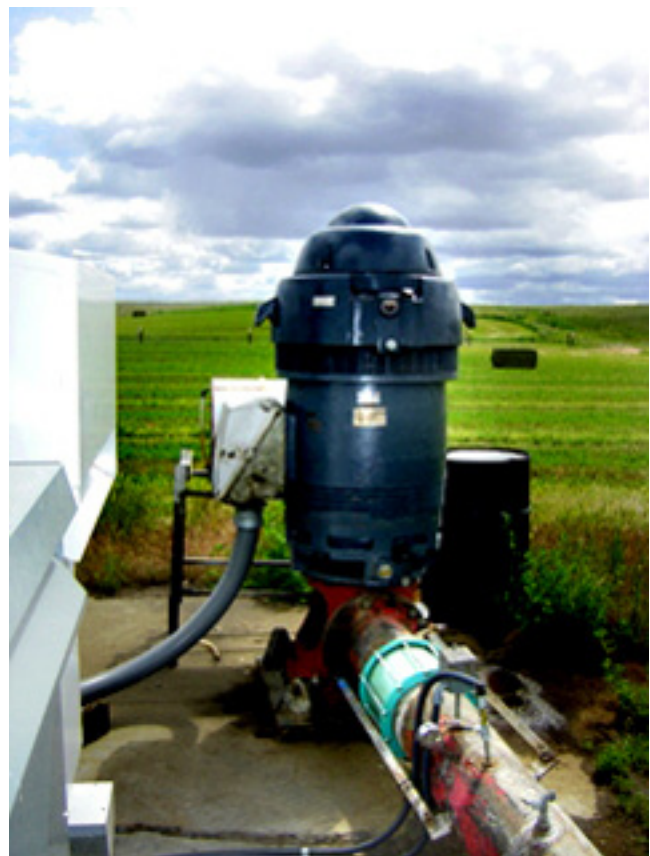
Figure 12-31 Water well pump powered by electric motor, Washington
