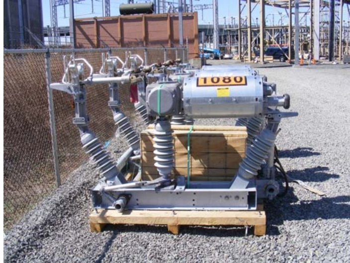
Fig. 9 - 26 kV 1200A Circuit Switcher for Capacitor Banks Shunt Reactors
