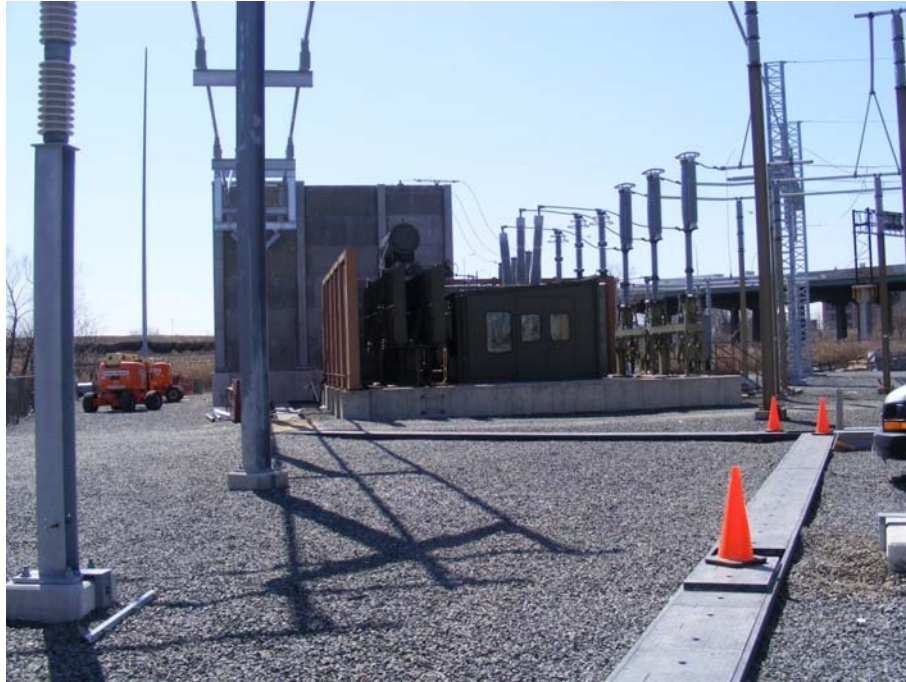
Fig. 12 - 230 kV Shunt Reactor Voltage Regulation
