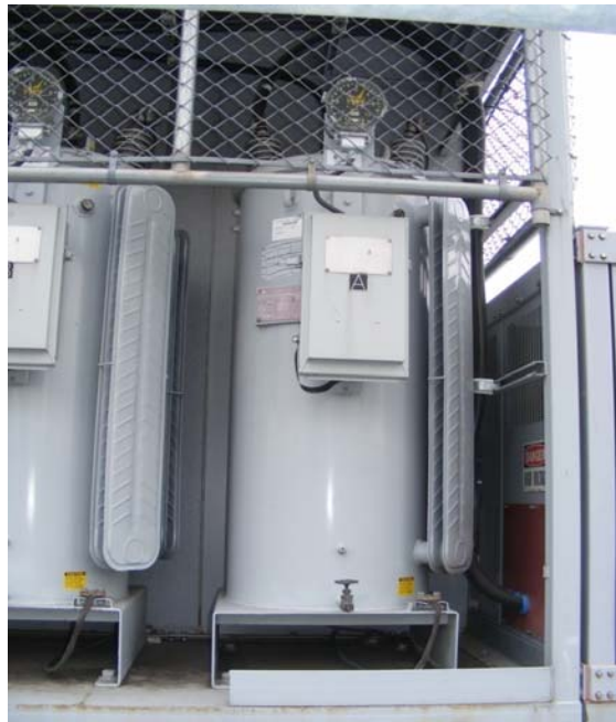
Fig. 14 - 4 kV Voltage Regulators
