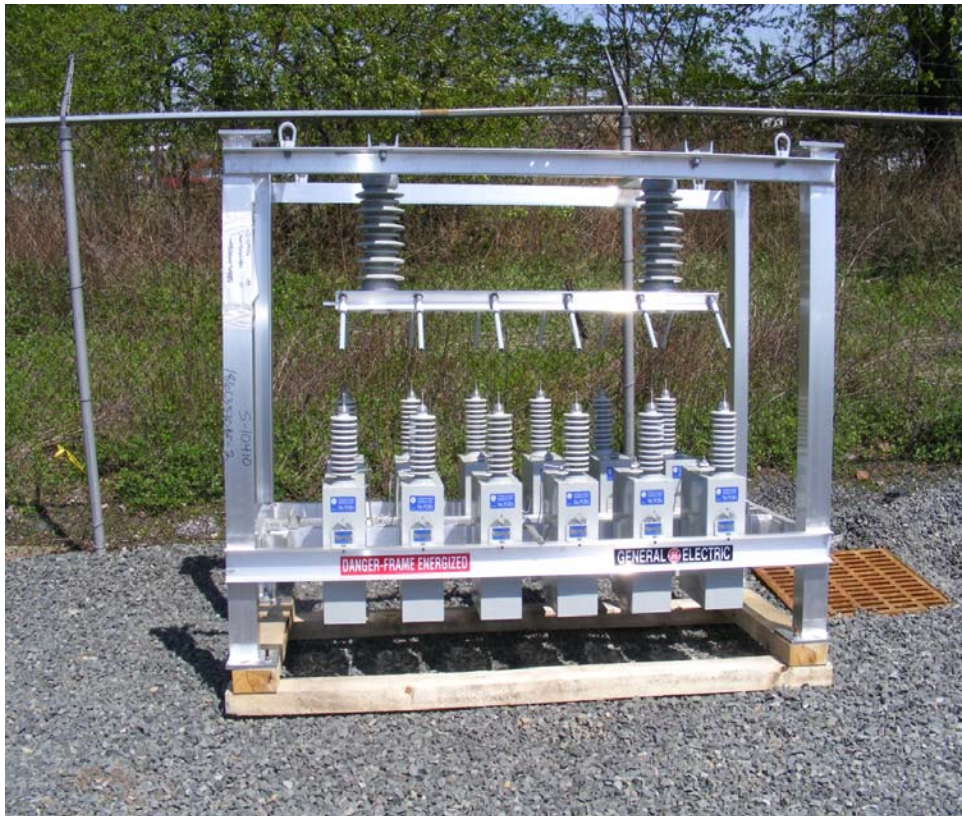
Fig. 4 - One Phase of 26 kV Capacitor Bank
