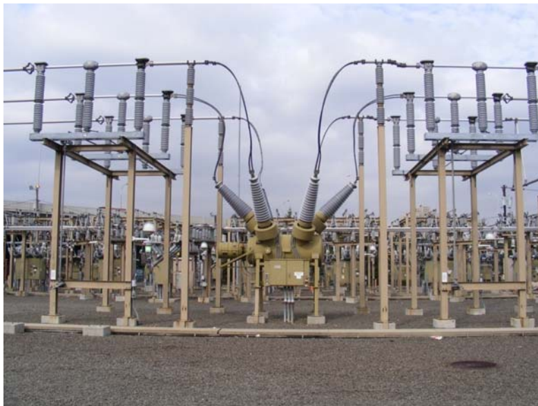
Fig. 8 - 230 kV 2000 A Circuit Breaker
